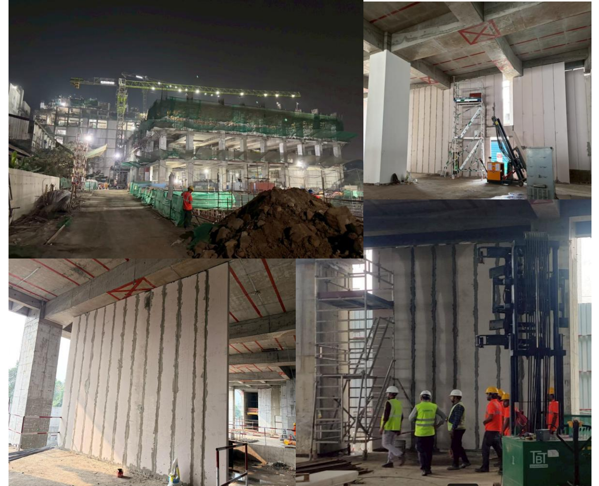
Data Center; Mumbai
