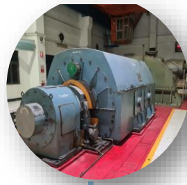
Waste Heat Generation (WHG)
